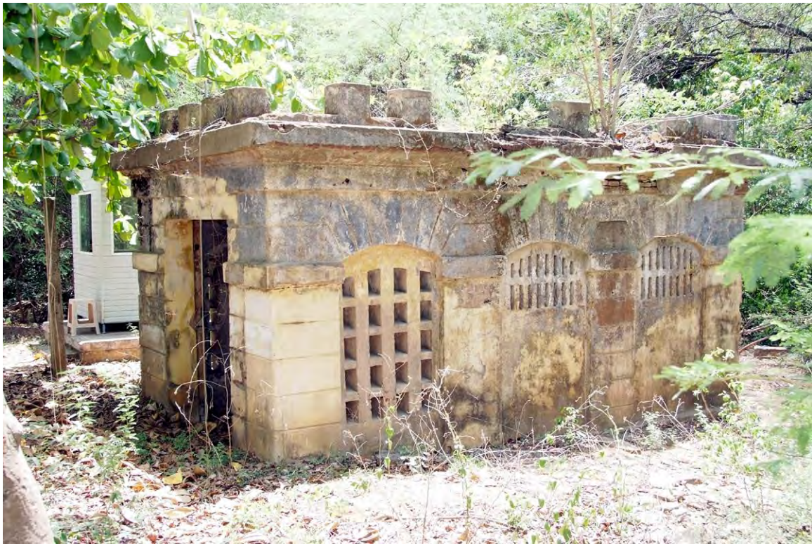
Below Taramani Guest House, the Mystery Structure of Trail One, as it appeared around 2010. Photo: P. Senthil
